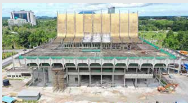
Ongoing Project of the Architectural, Structural and Civil Works for the Proposed Transformation of the State Legislative Building, Sarawak (SPAC)
