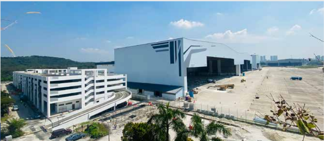
The Refurbishment of Main Building and Infrastructure Works at Subang Engineering Complex A, Sultan Abdul Aziz Shah Airport (SECA)
