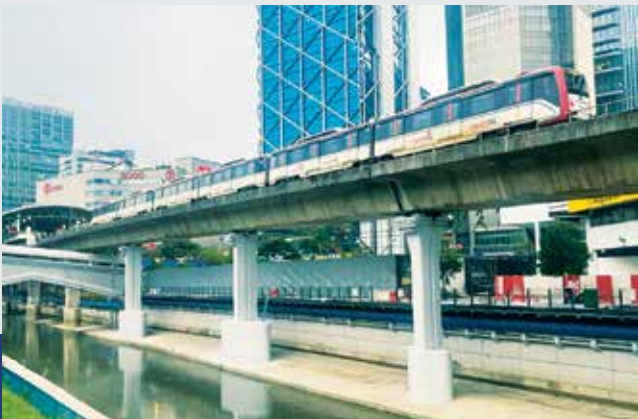
The Remedial Works at Pier 163 to 165 near Bandaraya LRT Station (P163) for Prasarana Berhad
