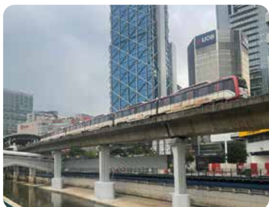
The Remedial Works at Pier No. P163, P164 & P165 and Associated Works near Bandaraya LRT Station of Ampang Line
