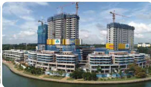
Residential Towers, Podium Block, Facilities Block, and Serviced Apartment on Plot 8MD3, Precinct 8, Putrajaya
